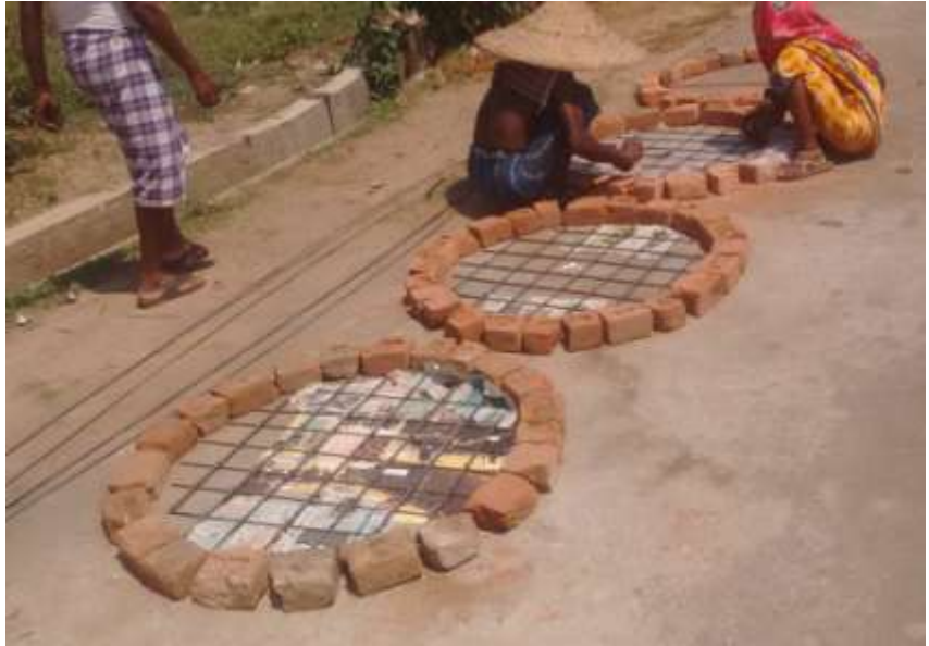
Pic 11: Mason making leach pit covers on the road near a toilet build.
