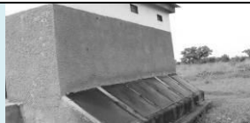
ECOSAN latrine in Alune P/S Akwang Sub County
