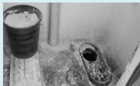
Inappropriate use of ECOSAN in Lumule P/S Kitgum Matidi Sub County (urine pipe blocked with faeces and ashes)
