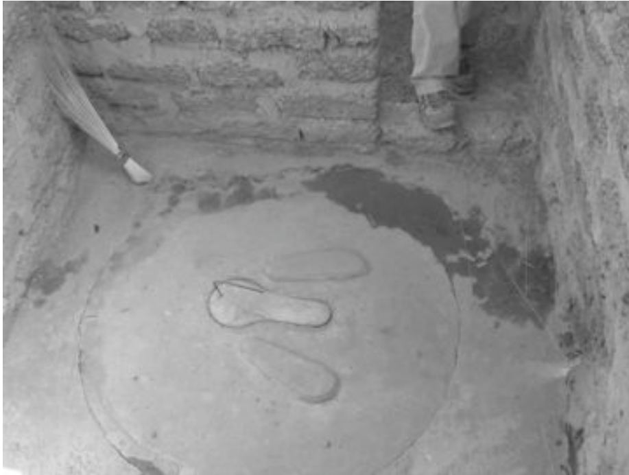
Figure 1.6 Sanplat latrine platform promoted by World Vision Mali's WASH programs.
