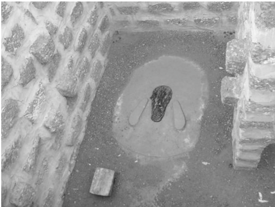
Figure 6.11 A latrine prototype using the design depicted in figure 6.9. Note protruding bricks to facilitate lowering to and rising from a squatting position, with a bathing stool in the foreground. Drainage under the enclosure wall is located just outside the photo on the left wall, just below the bathing stool. (Note that this prototype uses laterite brick and cement mortar. High quality clay can also be used for effective mortar with laterite brick, for considerably lower cost.)
