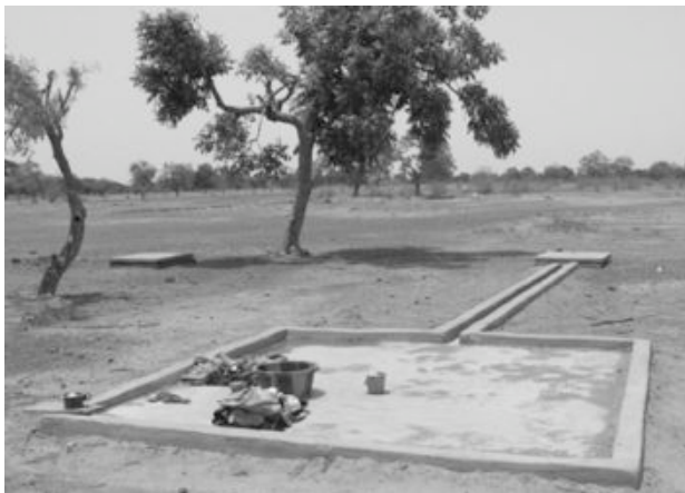
Figure 1.5 A typical laundry apron, usually placed within a few meters of the pump, which provides a convenient and hygienic place for clothes washing.
