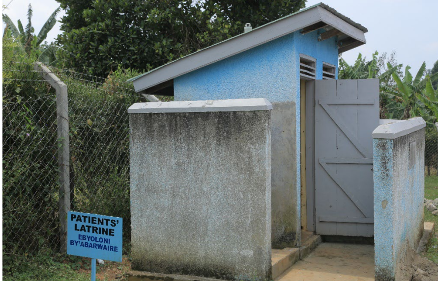
A traditional pit latrine for all patients at a health center III in Kabarole. The pit is not lined and will not be emptiable when it is full.
