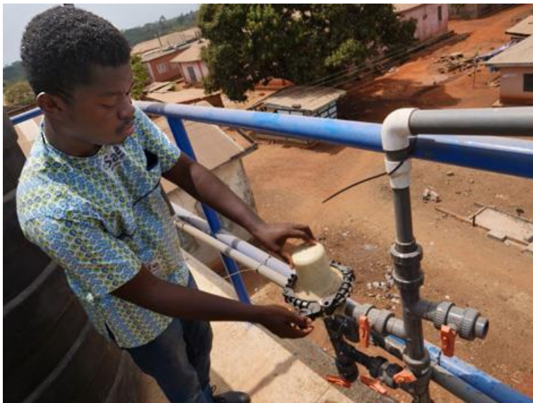
Martin Agyepong Safe Water Network field services officer checks a filter on the water tower at Wamahinso.
