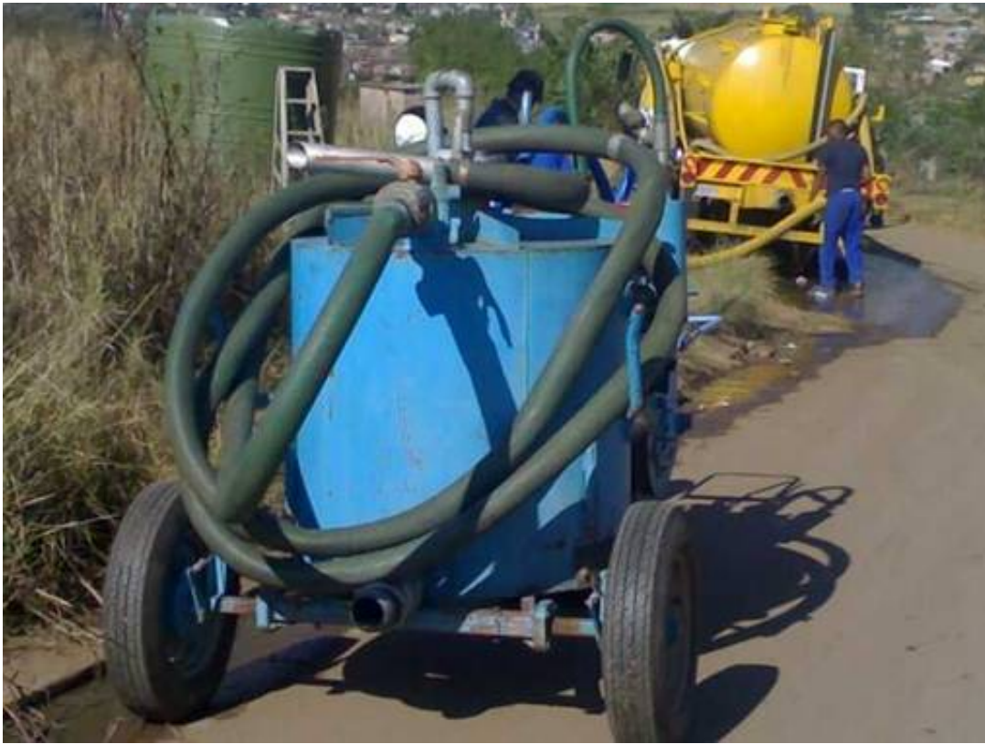
Figure 4: Vacutug, transfer tank and municipal vacuum tanker in Slangspruit, Pietermaritzburg
