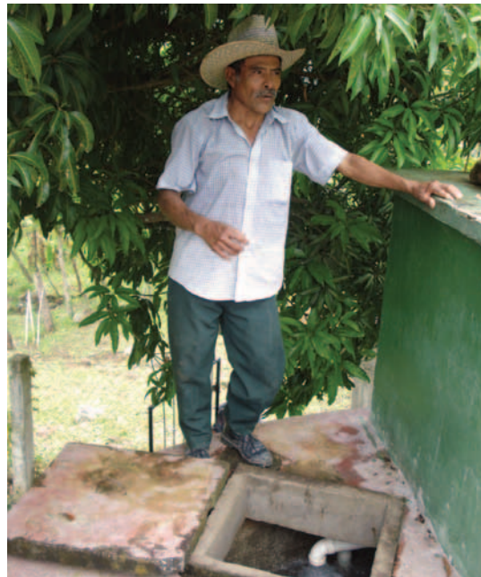
Eulalio Hernández, plumber of the community of El Tule, explains the steps in cleaning a tank.
