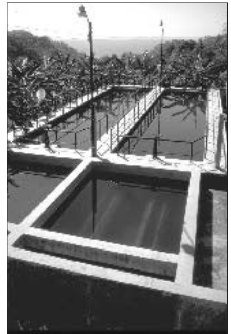
A small-scale wastewater treatment plant in Colombia. Credit: WHO photo library
