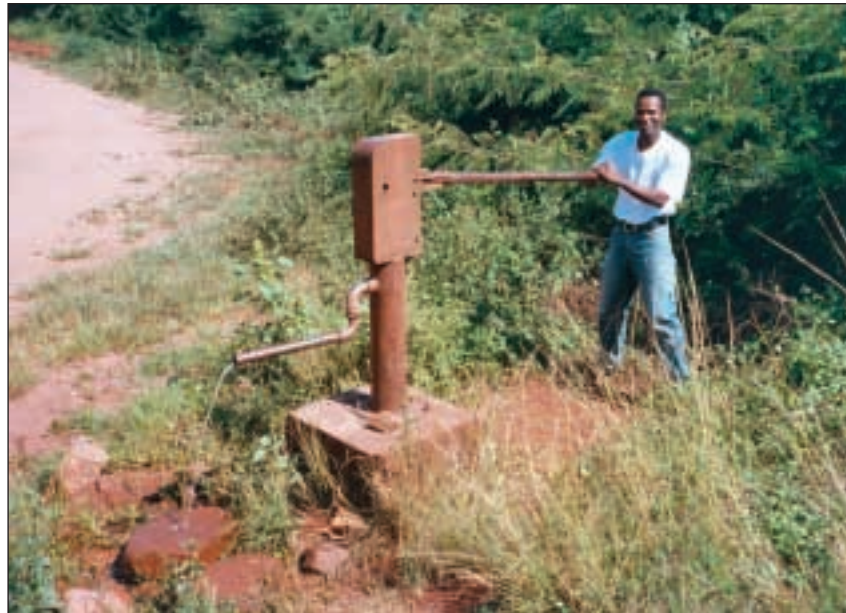
Plate 4) A working groundwater pump near Gogogo, South Africa. © Rob Hope
