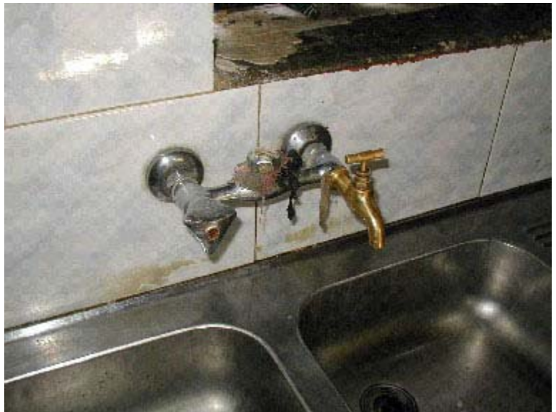
Photo courtesy of the WEPIA Program In the Mkhebe Foga village, 15 homes were retrofitted with new faucet fixtures to repair leaks.
