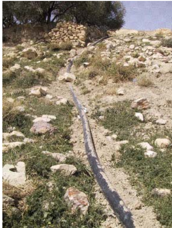
Photo courtesy of the WEPIA Program To reduce the amount of water lost in degraded cement canals used for irrigating orchards, 2,000 meters of plastic piping were installed in the place of the canals and covered with sand. This new system increased delivery and availability of water.
