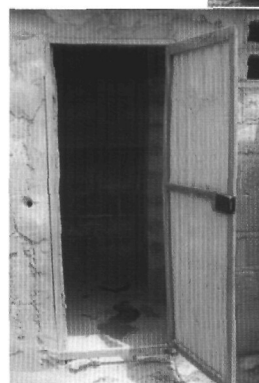
Rehabilitated traditional latrines in a planned peri-urban area.
