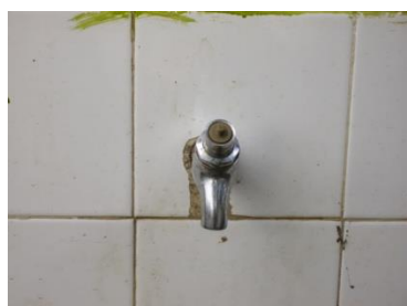
Figure 8 Tap does not work
