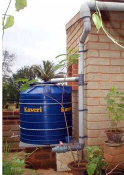
Figure 3: Basic system design; a basic rainwater harvesting system, such as the one pictured above, can be built of basic materials for the equivalent of $60, depending on local costs and system size; the main technical requirements are an impervious roof and room for a cistern or tank (Photo: S. Vishwanath, Rainwater Club).
